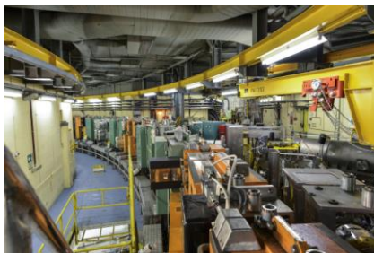
Inside the PS Booster © CERN
